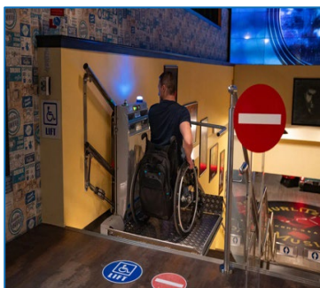
Photo 4 - stair platform lift
