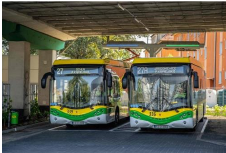
Figure 34: Buses charging at the transfer centre - Source: MZK Zielona Góra materials
