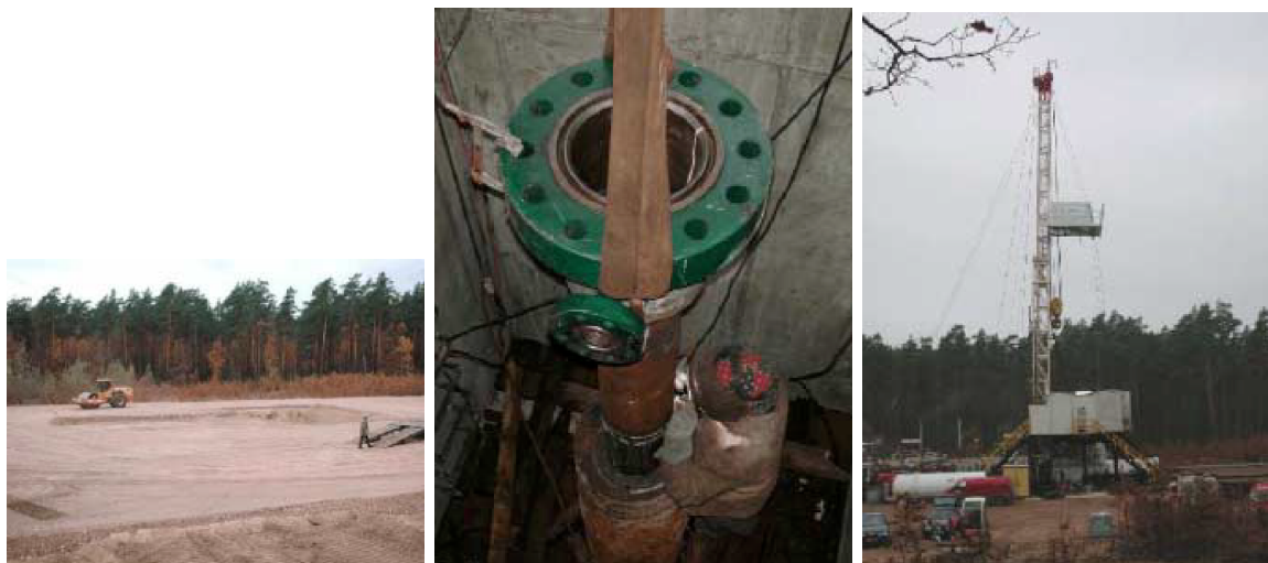
Figure G.3.11: Preparation of the drilling site (left), installation of a new casing head housing on top of the 10 years-old casing (middle), drilling rig (right).
