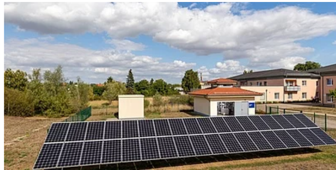
Figure C 9: Photos of the surface installation in Prenzlau ( https://www.energie-experten.org/projekte/tiefen-erdwaermesonde-mit-waermepumpe-im-prenzlauer-waermenetz ).
