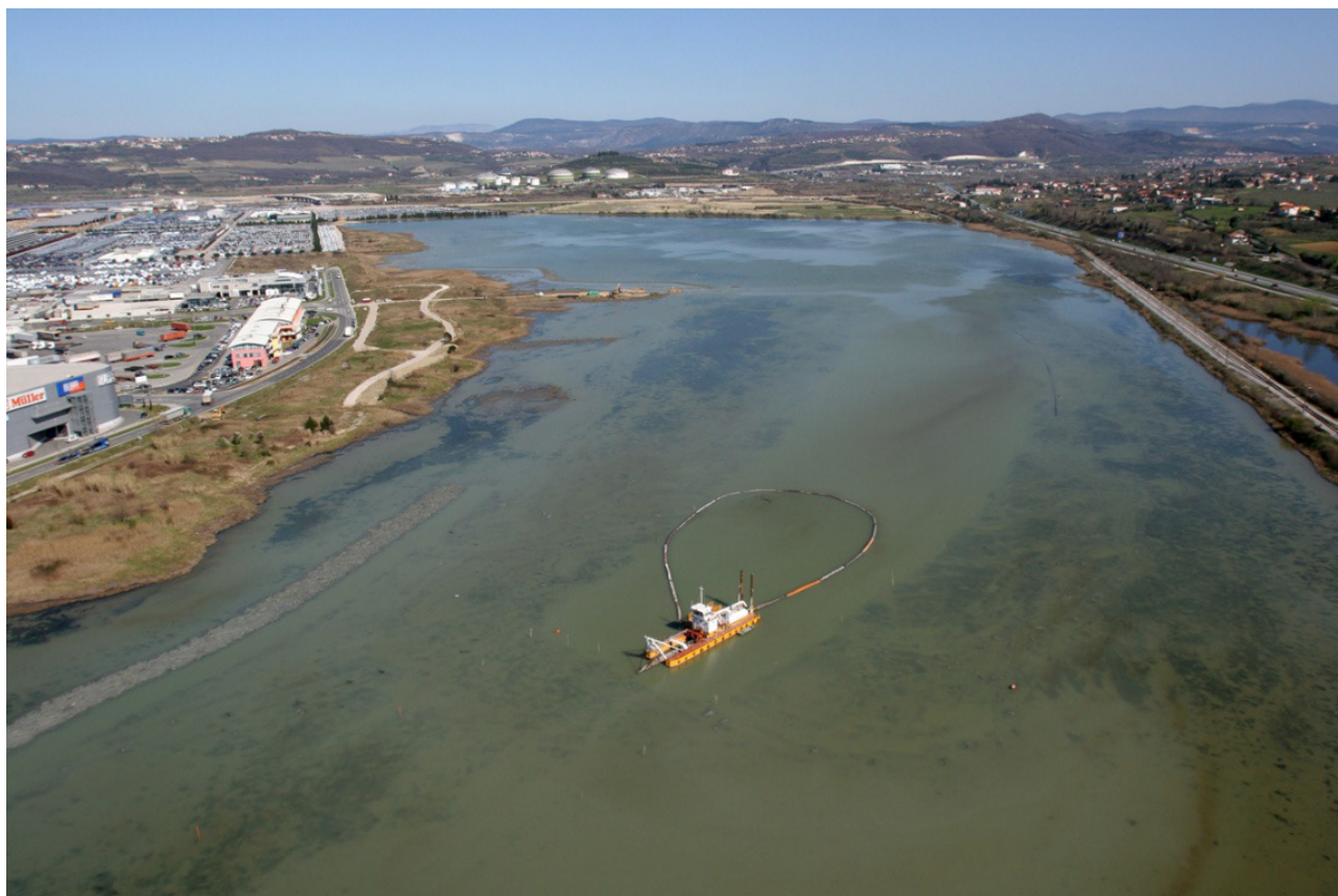
Removal of sediment and deepening of channels in the brackish lagoon in 2007 (NRSZ Archive).
